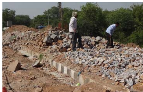
Rock splitters - not jailbirds - preparing the road - at 106F - all day long...
